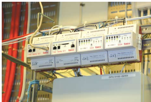
Access control and intrusion alarm is an integral part of TAC's delivery Integration and communication between climate and security systems is made possible through the Xenta 527
