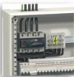
Stepped splitter block mounted on rail.
