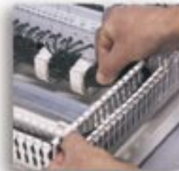
Associated with a vertical trunking, the wiring straps allow transparent and tidy wiring routing.
