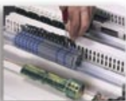
Feeders and earth are connected in spring loaded terminals.
