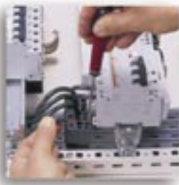
Connections are made using 6 mm 2 and 10 mm 2 tap-off terminals.
