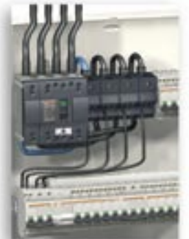
Polybloc 160 A distribution block supplied by NG160 circuit breaker.
