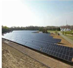
Power System Solution for Dayton, Ohio solar farm
