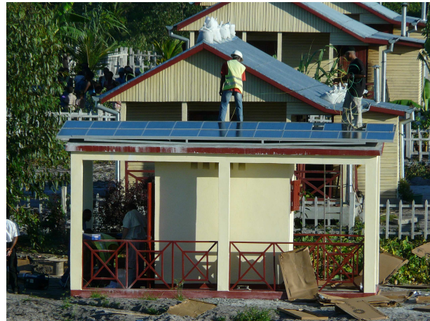
Schneider Electric's photovoltaic expertise being deployed in Marovato, Madagascar.
